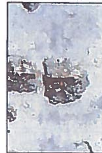
rotfend beton in dakopbouw
